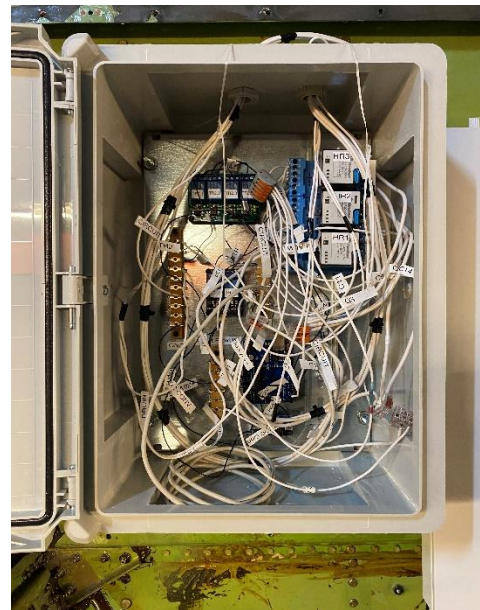
Figure 7 Junction Box Opened
