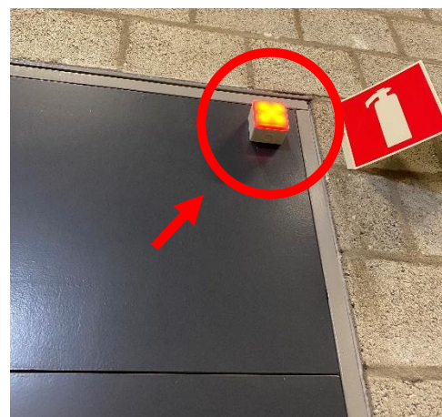
Figure 10 - RED LIGHT - Indication if generator ON or OFF - NOT GUARANTEED!!
