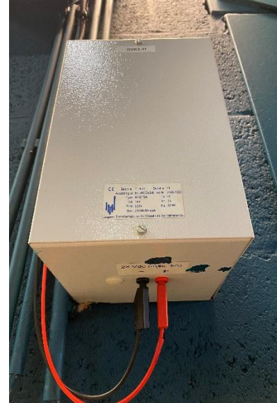
Figure 5 28V DC Power Supply
